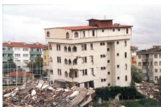
a) Collapse of the bottom floor
