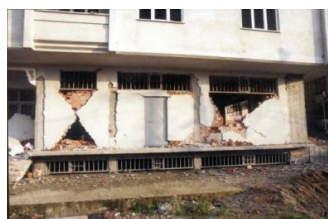
b) Moderate damage of the URM infill walls
